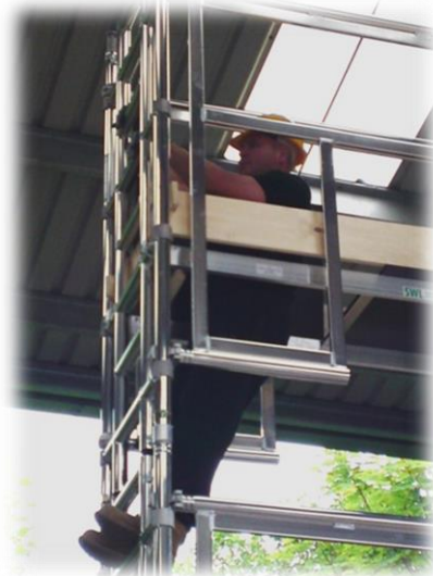
10. Access and egress to the next platform level through the trapdoor, using the ladder provided.
