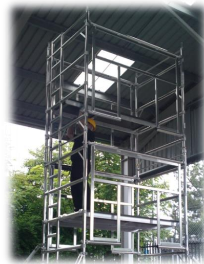
14. Remove the temporary trapdoor platform Position to the appropriate rung (Trapdoor facing the ladder section) 1 rung above the bottom section of the AGR frames.
